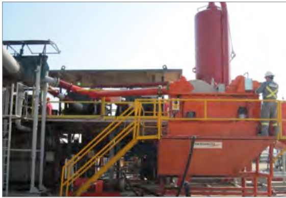
Figure 3: MD-3 shaker installation for Costero 24 well.
